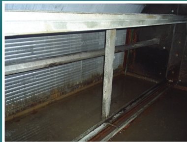
Air Handler Before UV Lights
