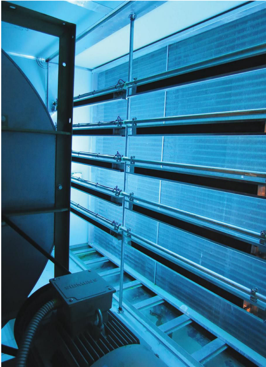
DISINFECTING WITH UVC: The APCO disinfection-odor control installed in the AHU disinfects and reduces odors with proprietary UV-C and carbon ceramic lifetime tiles. PHOTO COURTESY OF FRESH-AIRE UV
