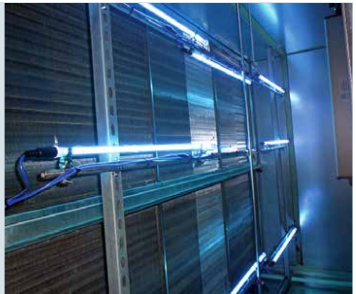
UVGI is effective for microbial disinfection of interior wall surfaces, coils and the supply airstream of air handlers
